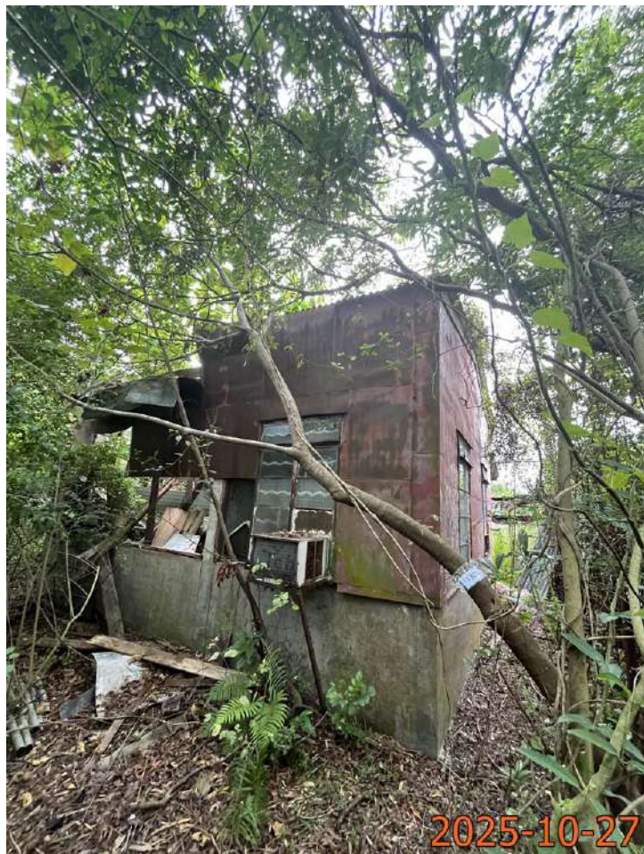
T30 (Overview) (Leaning)
